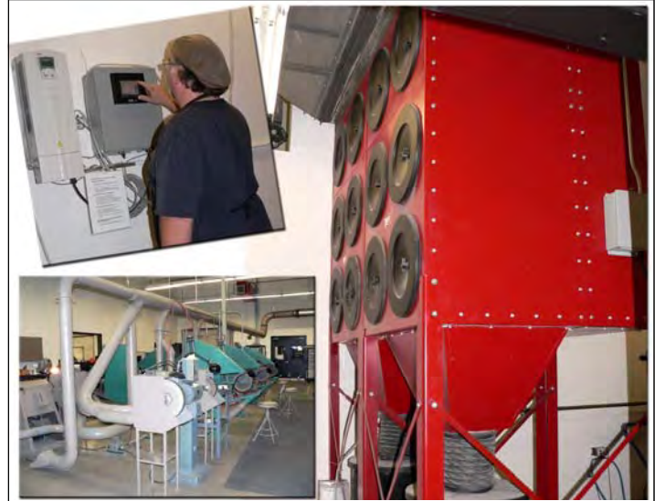
NIKE GOLF—Ft. Worth, TX. RP6-2 with Intelli-Touch Energy Savings Controls
