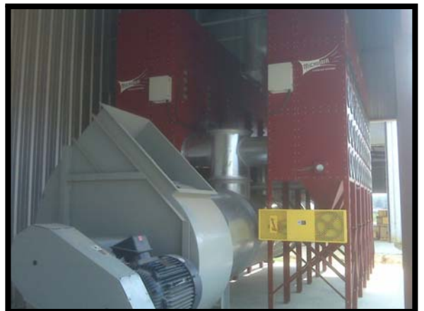
Tight Intake/Exhaust Ducting with Drop-Out Tees, Connected to a 60,000 CFM Blower
