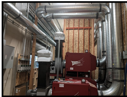
MX6000 Filter Room
