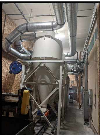
Cyclone Room for Chip Drop-Out
